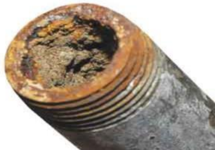
Example of galvanized piping
