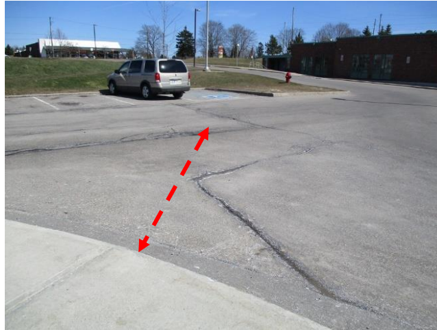
No curb ramp
