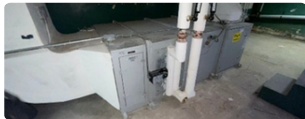
Air Handling Unit (AHU) with heating coils
